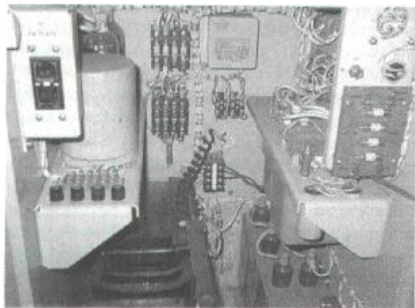
The massive power supply takes up the bottom half of the cabinet.
