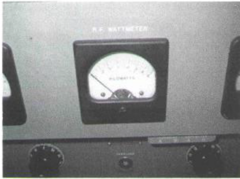
A 5 KW Wattmeter on the front panel !!!!
